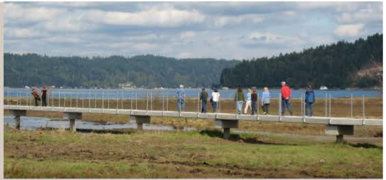
The WRIA 16 Planning Unit traverses the new walkway (still under construction) during a visit to the Skokomish River delta.
